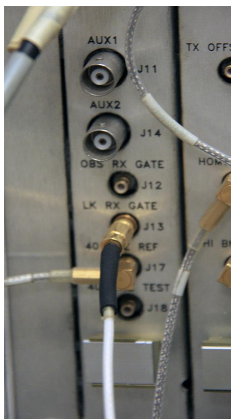
Figure 2. Junction board. J13 is Connected to the oscilloscope.
